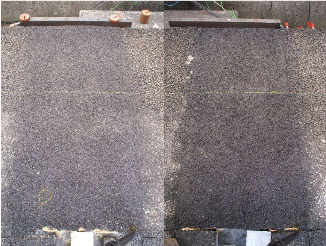
Figure 3. View on the two Prefab Silent Joint systems installed in the LINTRACK facility before trafficking. Left: closed joint, referred to as joint -13 mm. Right: opened joint, referred to as joint +13 mm.
