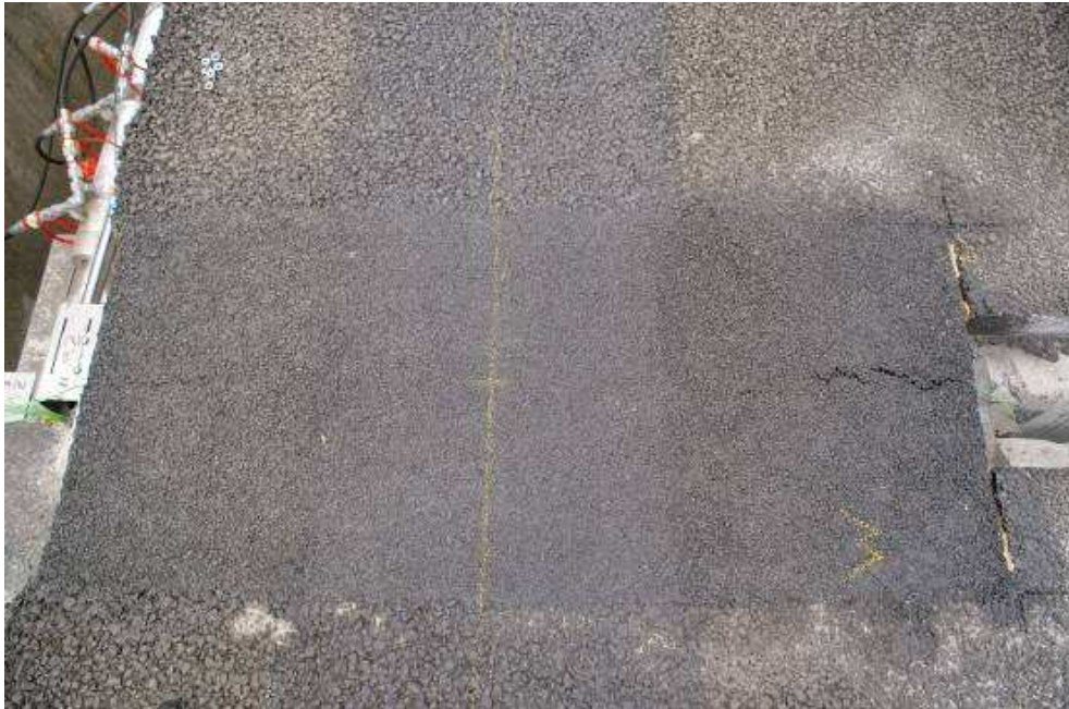
Figure 31. The +13 mm joint at visual failure. A crack develops at the left edge of the joint exactly above the built-in temperature gauge. The crack at the right edge first appeared after initial joint opening.
