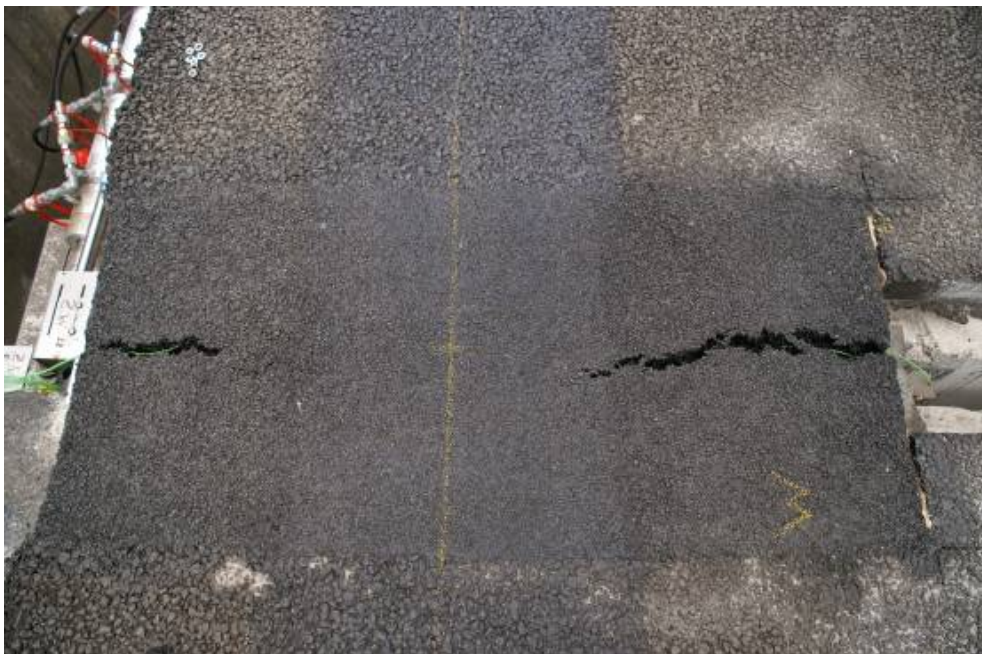
Figure 32. Impression of the +13 mm joint after failure.
