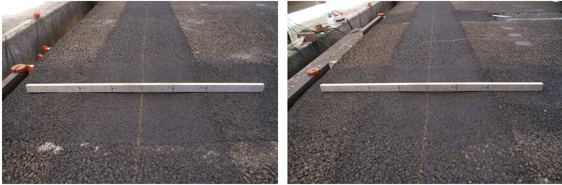
Figure 21. Rutting in the Prefab Silent Joint after 85,000 load repetitions. Left: +13 mm joint, right: -13 mm joint. (also see Appendix C)
