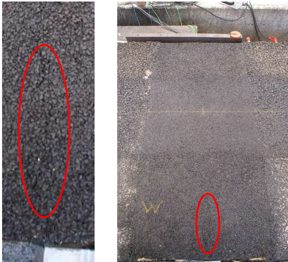
Figure 4. Surface defect in +13 mm joint before trafficking (left) and at the end of trafficking (right).
