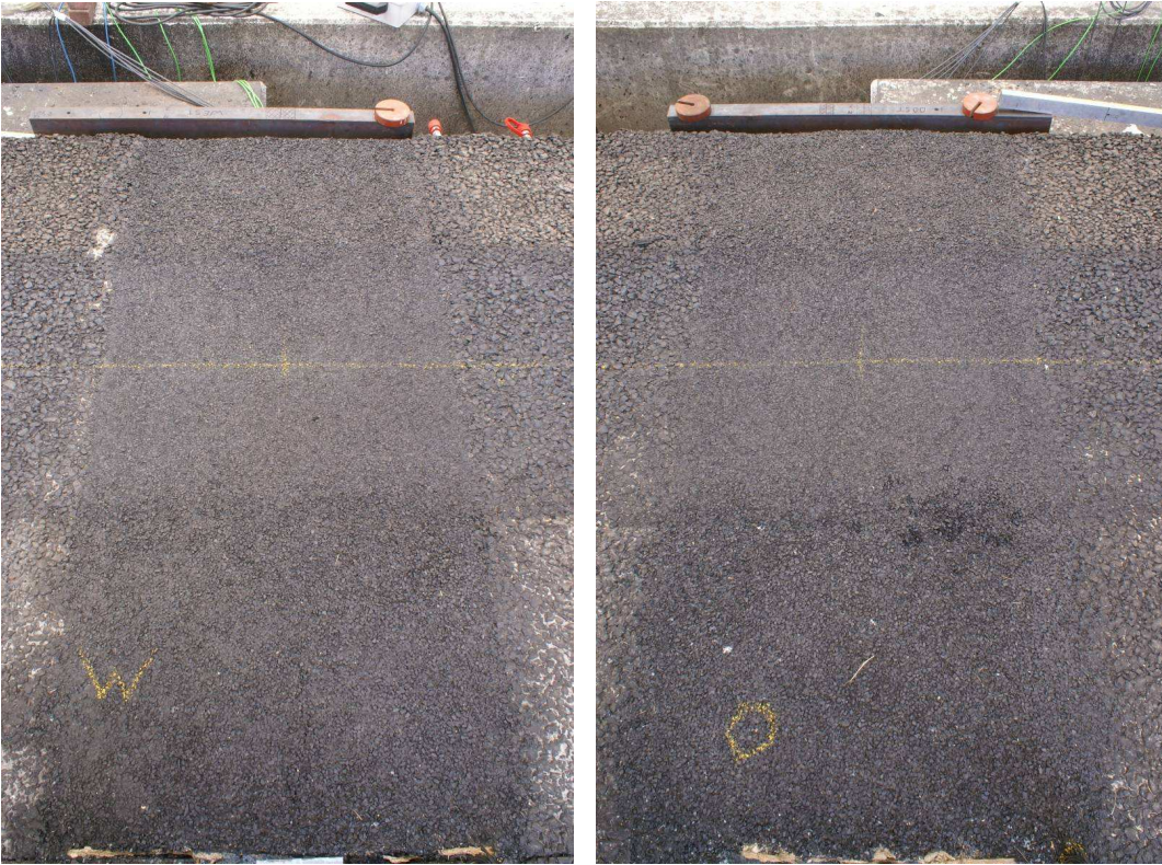
Top view at N=85000. Left: +13mm joint, right: -13mm joint.
