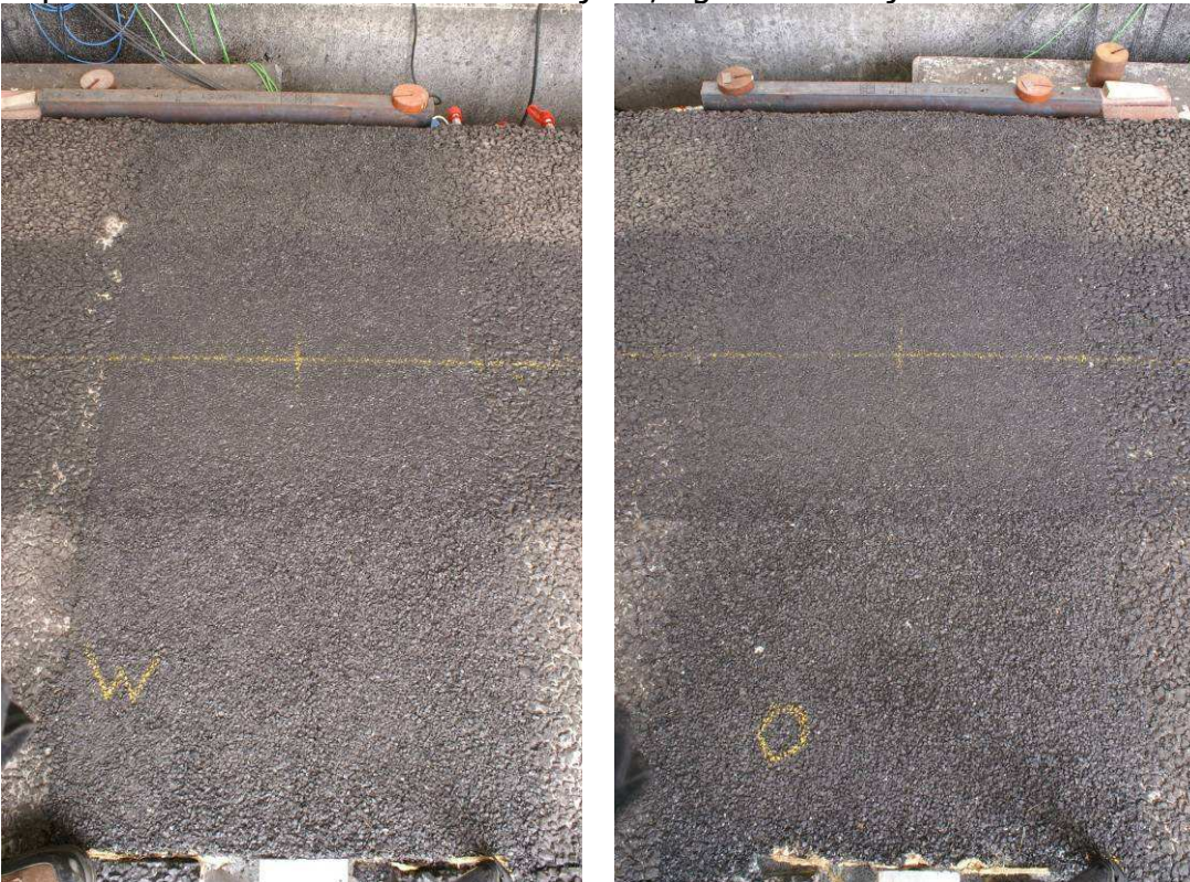
Top view at N=80000. Left: +13mm joint, right: -13mm joint.
