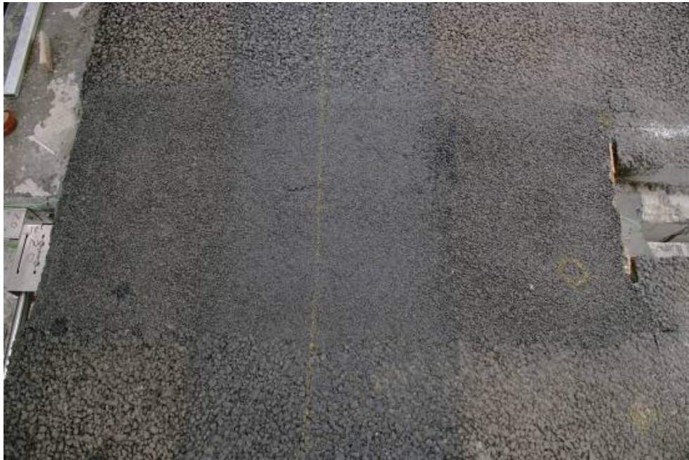
Figure 29. The -13 mm joint just after visual failure. A crack develops at the wheel path centre exactly above the joint between bridge and bridge support.
